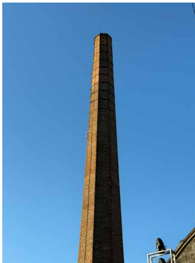
Fig.52 Chimney photographed in 2024
